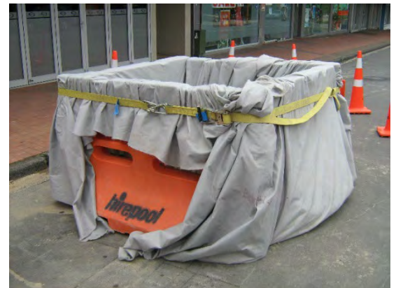
Figure 107: Example of a mobile 'turkey nest' used for dewatering
