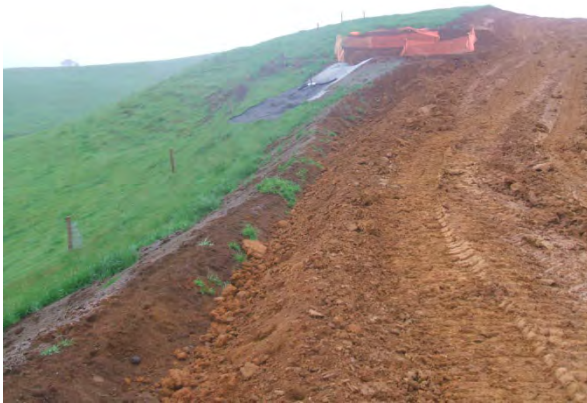
Figure 124: Decanting earth bund and diversion bund installed during a farm track construction
