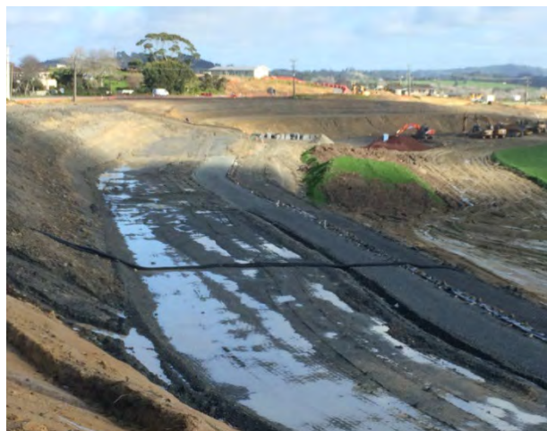
Figure 34: Pipe-drop structures conveying upper water down an exposed slope
