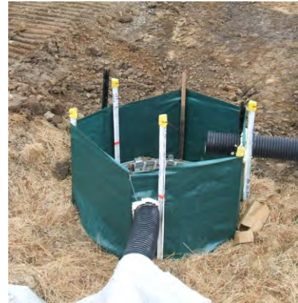
Figure 98: Good use of a silt fence installed to protect a new stormwater catchpit where impounded water will not create a flooding hazard
