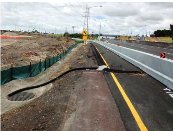
Figure 18: Hotmix bund diverting the motorway runoff to the catchpit
