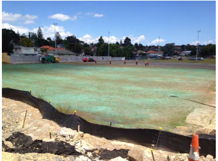
Figure 49: Sports field being hydroseeded. Sediment control remains installed until an 80% grass strike has established
