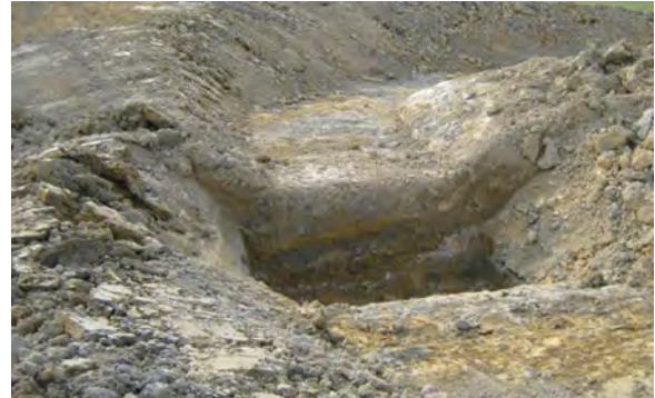
Figure 21: Drop out pit
