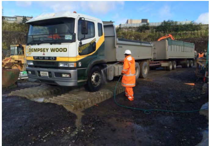
Figure 37: Example of truck wash and shaker ramp
